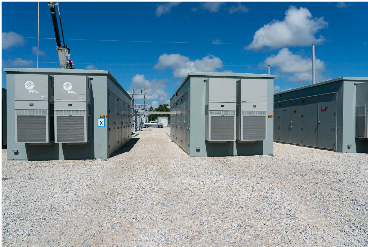
The Manatee Energy Storage Center in Parrish, Florida, is pictured on Aug. 12, 2021. North Dakota regulators approved two battery storage systems from NextEra Energy to be constructed near wind farms in Emmons and Burke counties. (Photo courtesy of NextEra Energy)
